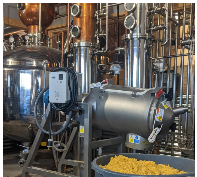
Figure 1. The Liquid Solid Separator™ is installed at Blue Valley Spirits to remove spent grains from ethanol
