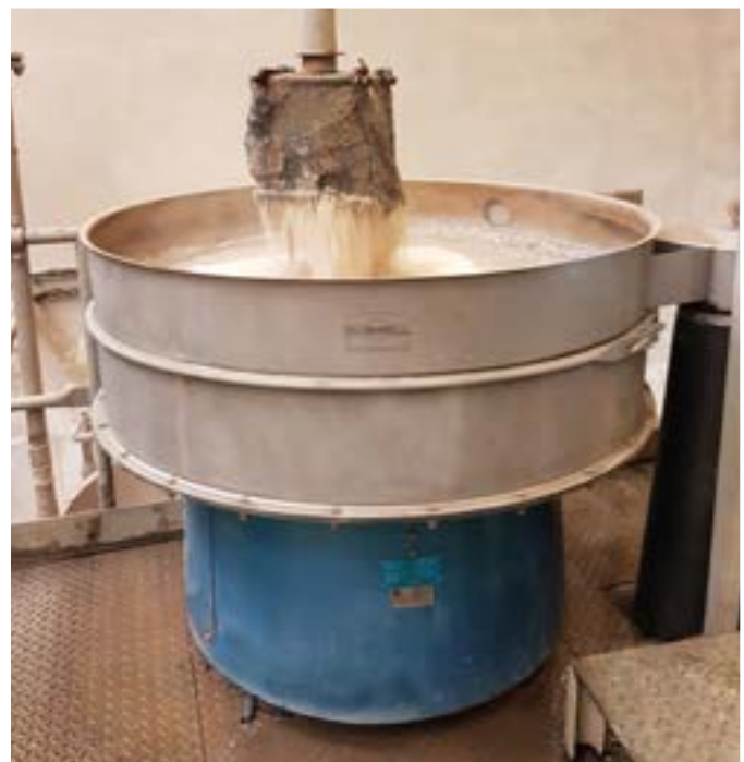
Figure 1. The Finex Separator™ is installed at PFR Nord to separate the solids from the wash water
