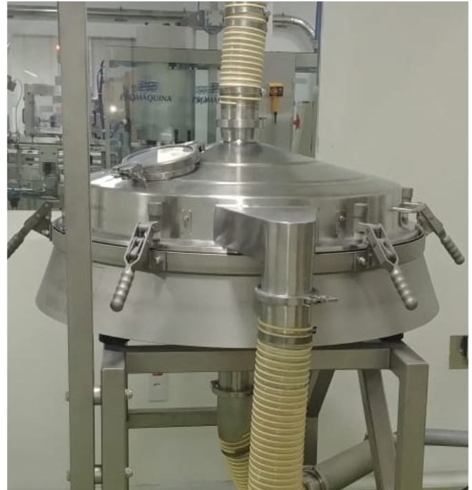
Figure 1. The installation of the Russell Compact Airswept Sieve™
