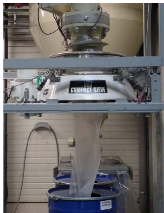
Figure 1. Installation of the Russell Compact Sieve® at Profel Extrusion & Finishing
