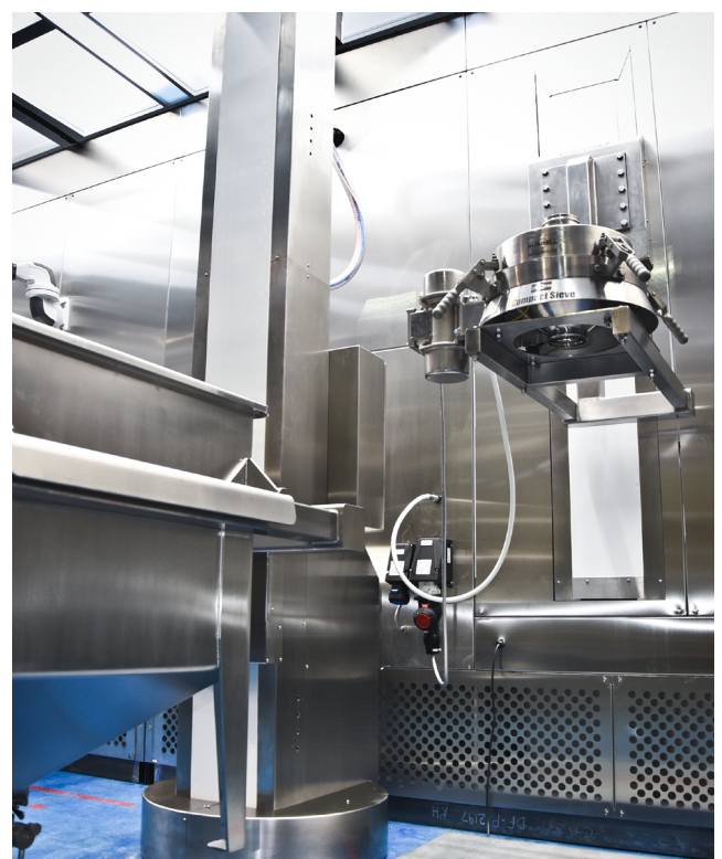
Figure 1. Installation of the Russell Compact Sieve® next to the elevated loading hopper
