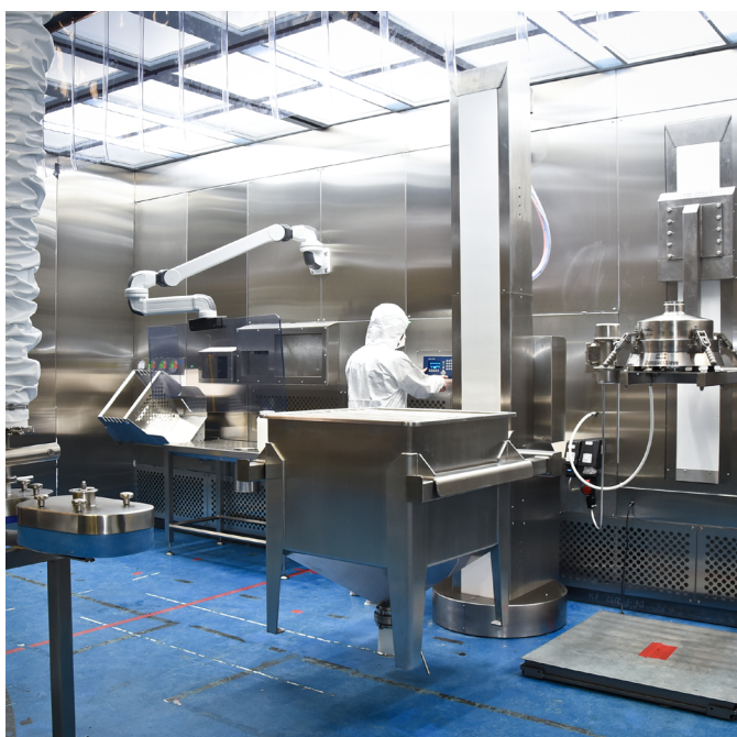
Figure 2. Installation of the Russell Compact Sieve® inside an ETL downflow booth
