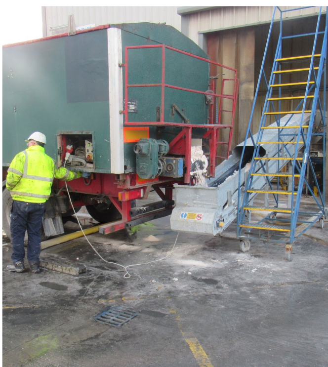
Figure 2. The Russell Compact Sieve® is used to screen up to 48 tonnes of incoming powders a day.
