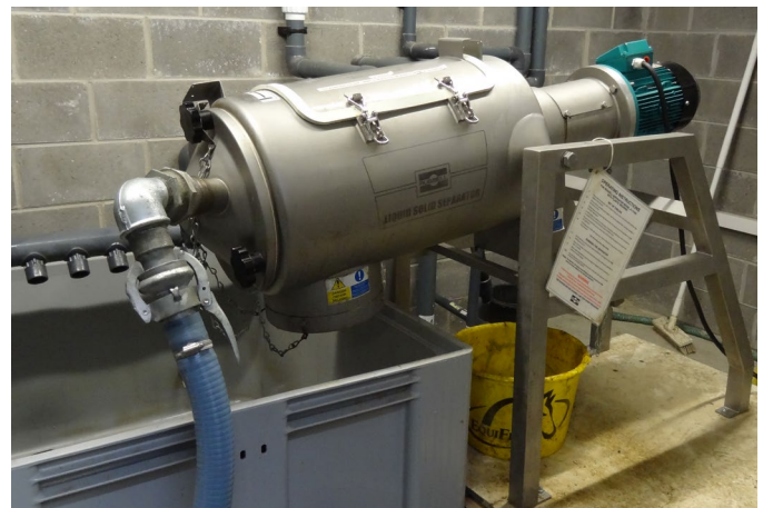
Figure 1. The Russell Liquid Solid Separator™ installed at horse rehabilitation centre to effectively clean wash water
