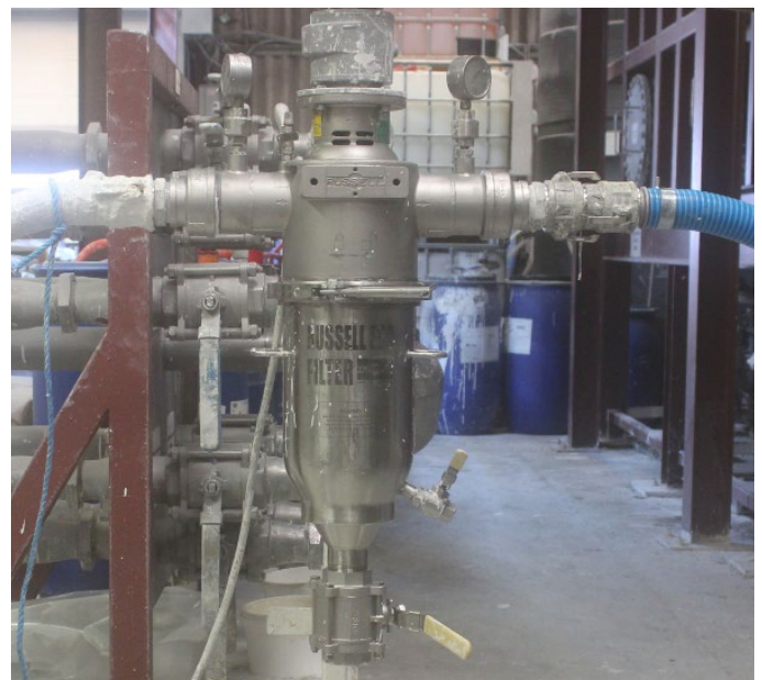
Figure 1. The Self-Cleaning Russell Eco Filter® is installed at Farrow & Ball to remove undispersed pigments of powder from paint.
