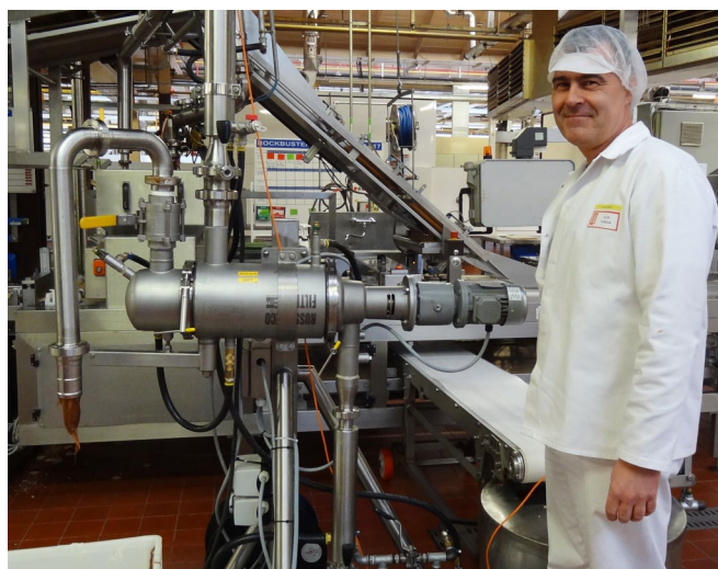
Figure 1. Self-Cleaning Russell Eco Filter® installed at the Mondelēz production site in Herentals, Belgium
