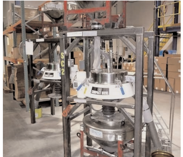
Figure 1. Russell Compact Sieves ® installed at the Deloro Stellite Plant in Indiana
